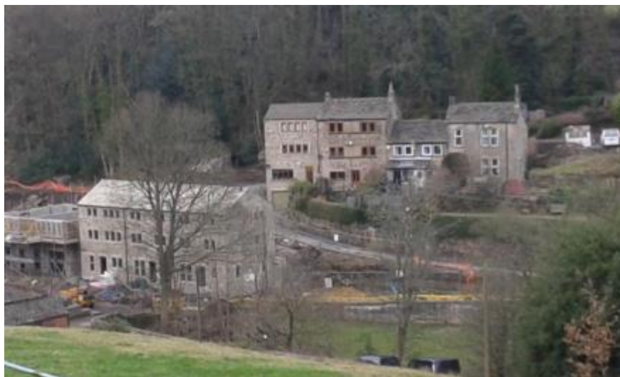
Figure 12 - New build homes being constructed to fit in with the local style, Upperthong
